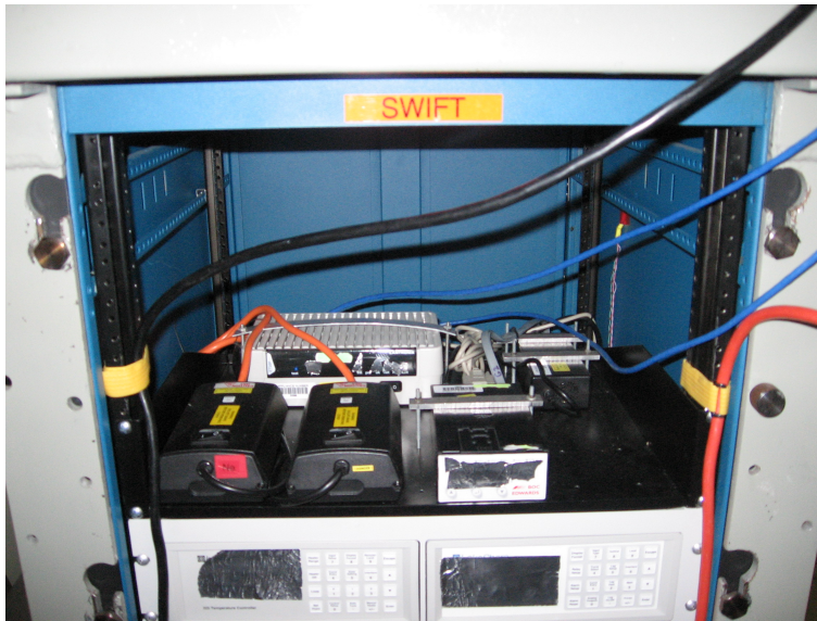
Figure 2: Top shelf of electronics rack with out cables. Showing Arc lamp power supplies, terminal server and pressure monitor. Power cables (orange and black) and network cables (blue) can be seen going off to connections on the other side of the cage.
