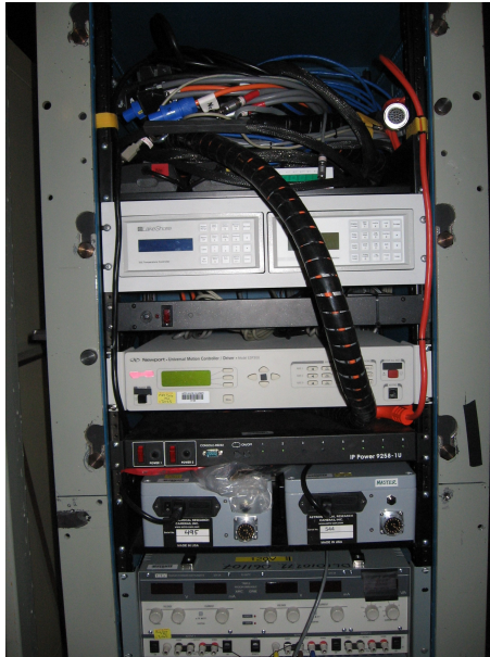
Figure 1: SWIFT electronics rack with umbilical cable coiled on top of upper shelf. From top to bottom, the electronics are 1) (under cables; see figure 2) Arc lamp power supplies, terminal server, pressure monitor, 2) Lakeshore 218 and 325, 3) Power strip 4) Motor controller 5) Network power supply 6) SDSU power supplies 7) general power supply
